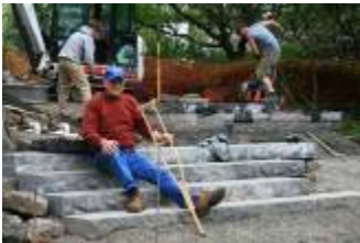
Bob MacArthur takes a moment away from supervising the construction at CSRG to rest his knee.
